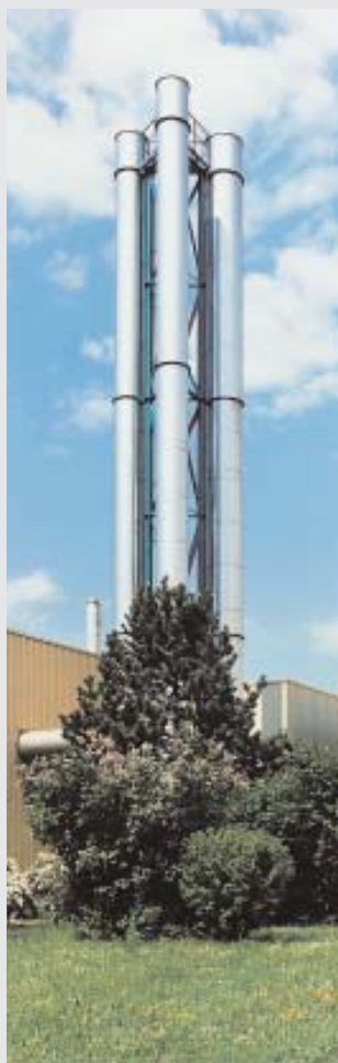
So far only the Wiesloch site has begun participating in emissions trading; it has a heating plant with an output of 28 MW.
